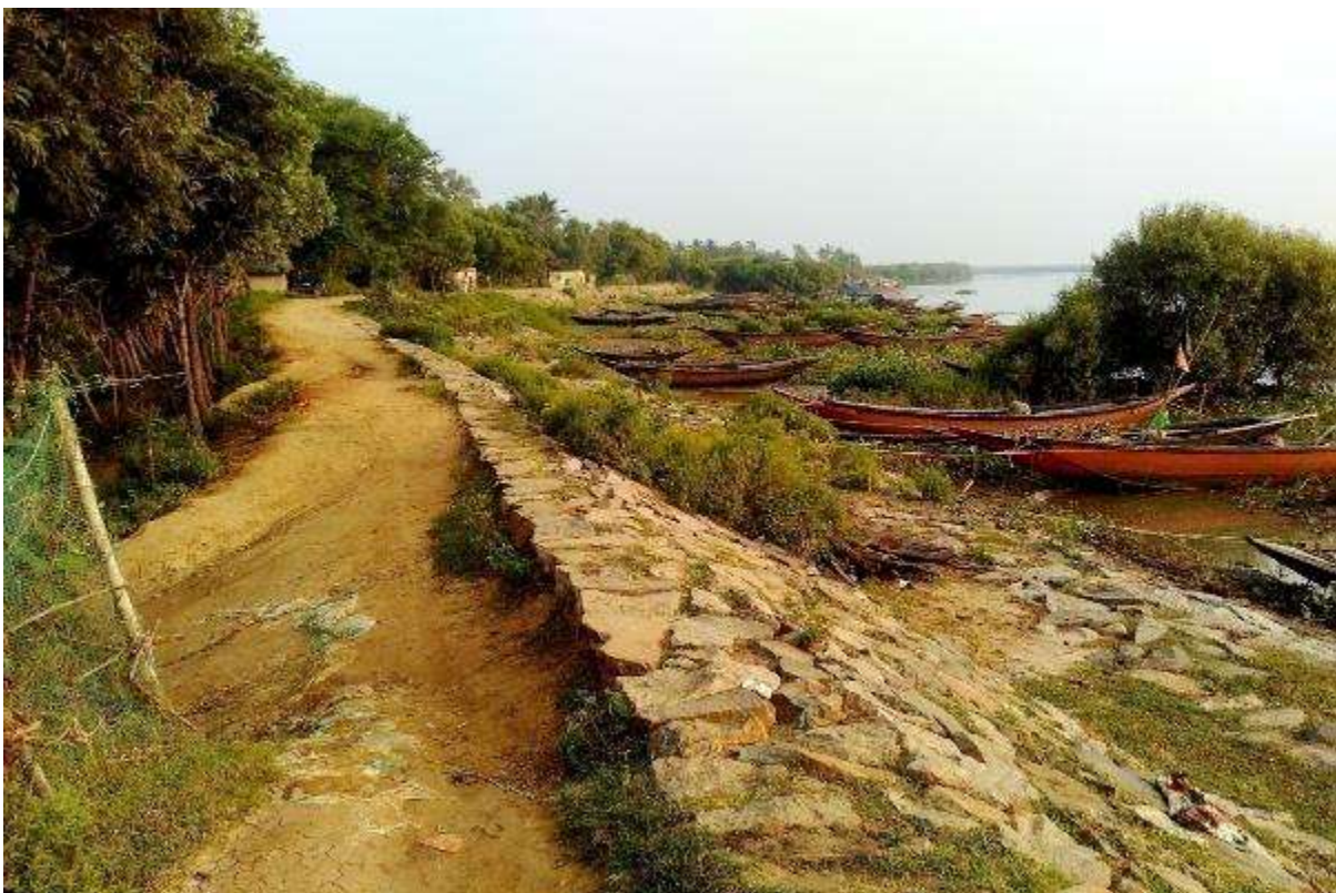
State of saline protection embankment in some pockets in normal times: Batighar area, Mahakalapada, Kendrapada district
